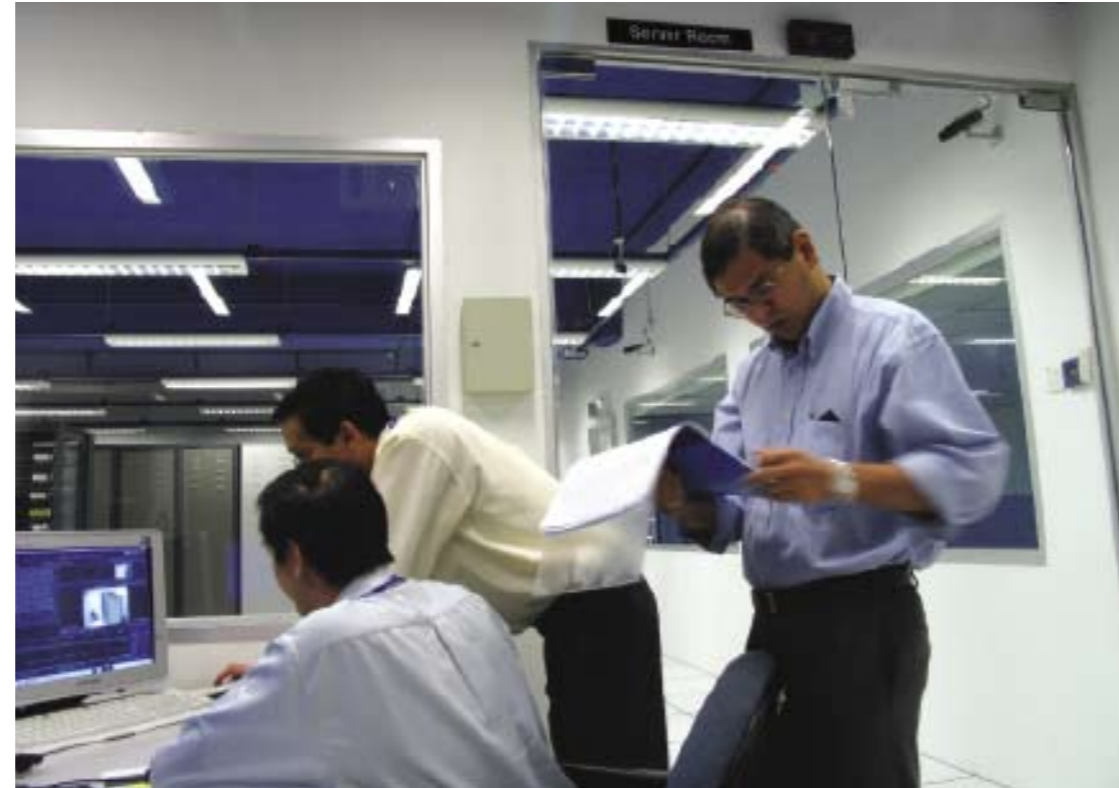
Other than the day-to-day operations and maintenance, the shared services in our Data Centre are complemented with our 24x7 SAINS Call Centre.
